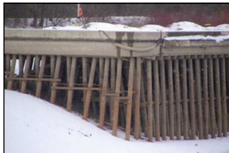
A typical pier construction is shown in this photo. Note the potential ambush areas underneath of the pier slabs
